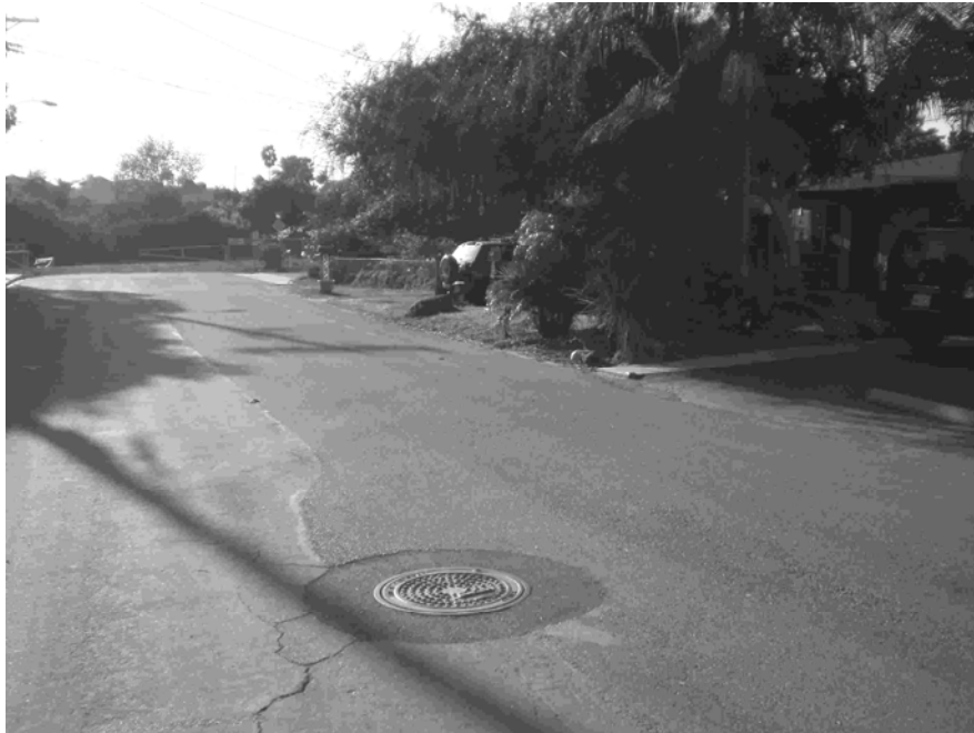
Figure 8. Site #4, in the City of Carlsbad, CA. Very shallow manhole (20" deep) with little warning of potential surcharge. There have been previous SSOs at this location.
